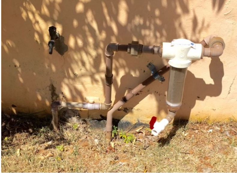
Photo 3: Drinking water filter in fill line to tanks in tower of Casa de Luz
